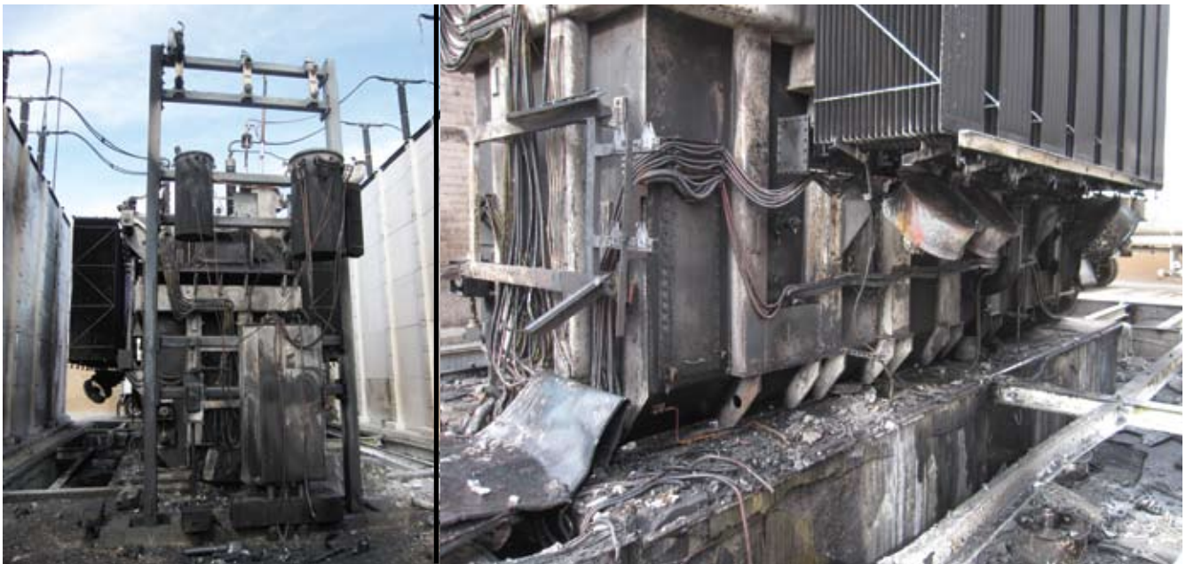
Front and side views of the burned unit with the tertiary structure beside it, although all the equipment on this structure was destroyed, NV Energy was able to repaint and put the steel structure back in service.
