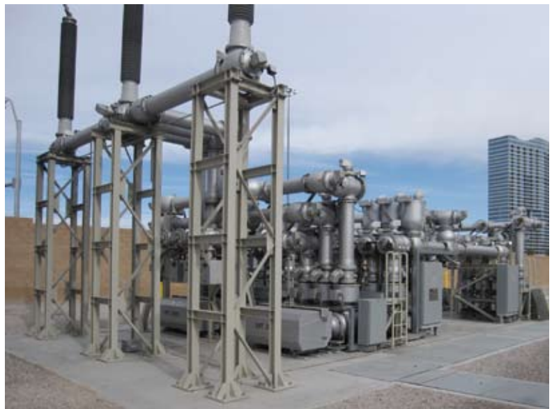
The undamaged 230-kV GIS equipment was protected by the firewalls.
