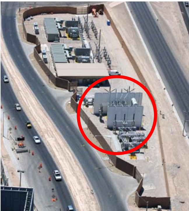
Aerial view of the entire Sinatra substation showing the location of the fire.
