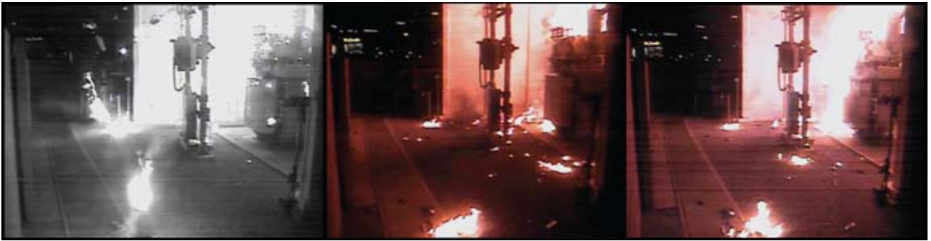
These are frames from the security camera in the Sinatra Station. Note how the first frame seems to be black and white, until the developing transformer fire starts to provide some more colorful lighting.
