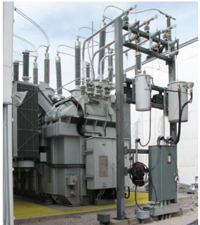
The 230/138-kV autotransformer tucked between the two ceramic panel firewalls before the fire.
